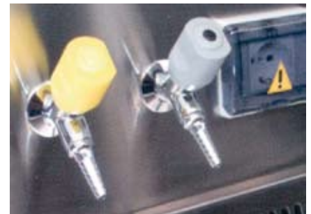
Cabinet services fixtures
