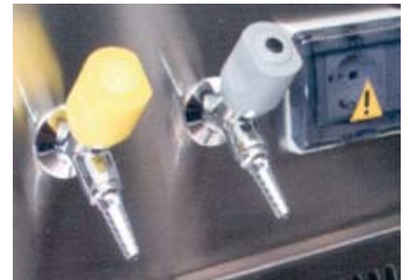
Cabinet service fixtures
