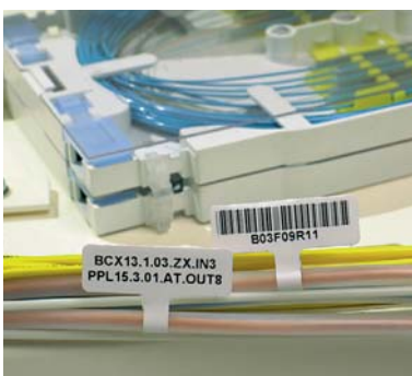
Fibre Optic Cable Markers
