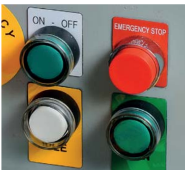
Control Panel Labels
