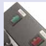
separate power and light switches
